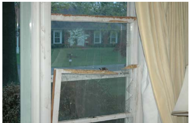
One of many windows damaged by the raccoon - the storm window made his attempt to escape a failure
